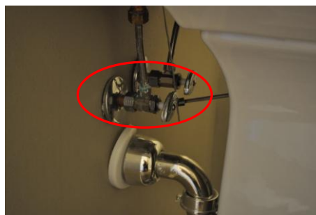
Corrosion build-up on the supply line in the lower bath. Recommend turning the valves once a year to prevent them from sticking.
