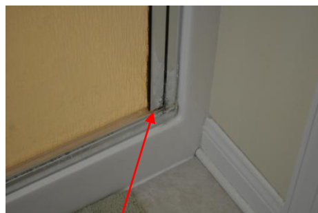
A little corrosion found on the bottom of the master bath shower door.
