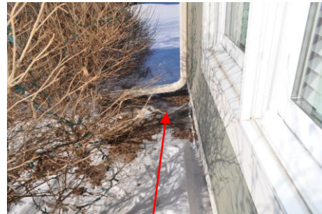
A low spot was observed on the SW corner of the house. Fill with black dirt so that you maintain positive grade.
