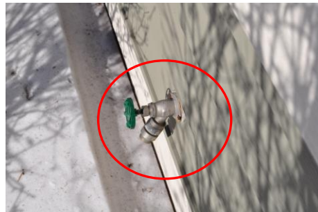
The outside hose bibs are shut off inside and they all have anti-siphon devices. Very good!
