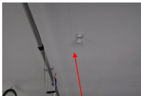
Shrinkage cracks located on the garage ceiling. Common with new construction.
