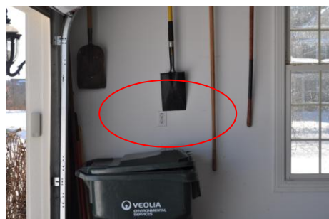
Two outlets in the garage trip the GFCI when I plugged my tester in. Recommend an electrician investigate.
